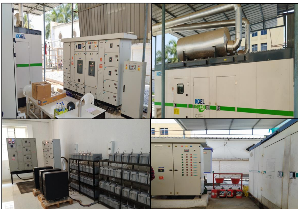
Energy conservation facilities observed in the Campus
