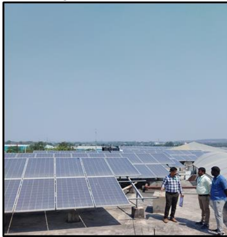
Solar Panel observed inside the campus
